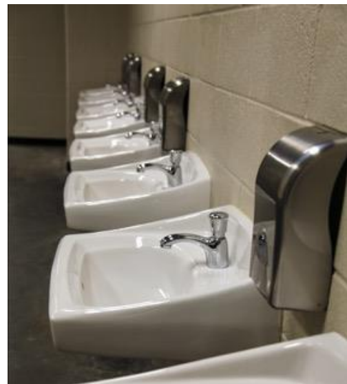
Lucerne wall-mounted sinks are paired with water-saving pillar tap metering faucets, all from American Standard, to outfit the public restrooms in the Atlanta Braves’ SunTrust Park.
