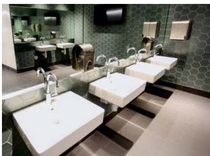
Single-handle GROHE Concetto bathroom sink faucets showcase sleek, slim design lines, along with water efficient performance, in the club-level restrooms at SunTrust Park.
