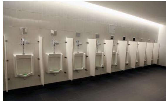
The WaterSense-certified Washbrook FloWise universal urinal and manual flush valve from American Standard operate in combination to provide water efficient performance using only 0.125 gpf.
